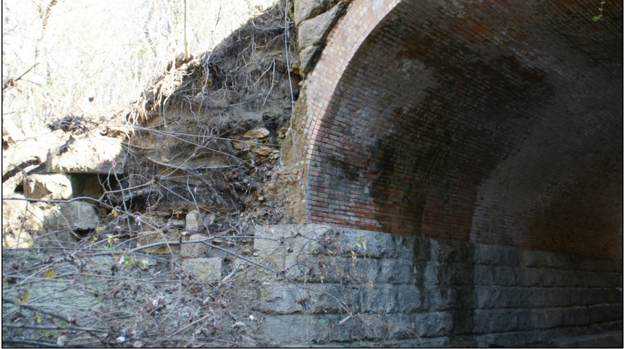
Upstream Block-Wingwall on the left has failed.
