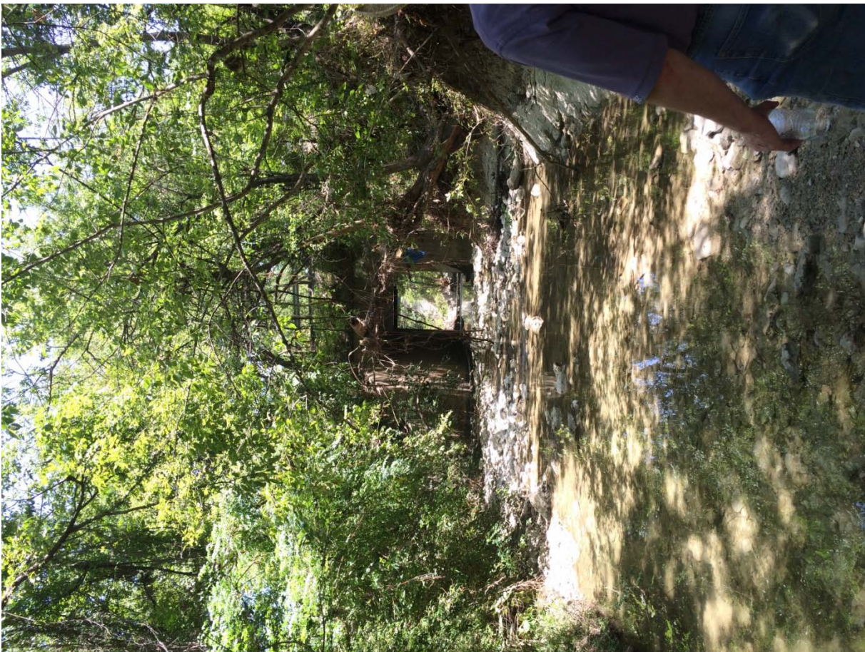
Looking downstream/1 barrel box culvert with wing walls/There is an outlet pipe to the left of the top left corner of the box culvert
