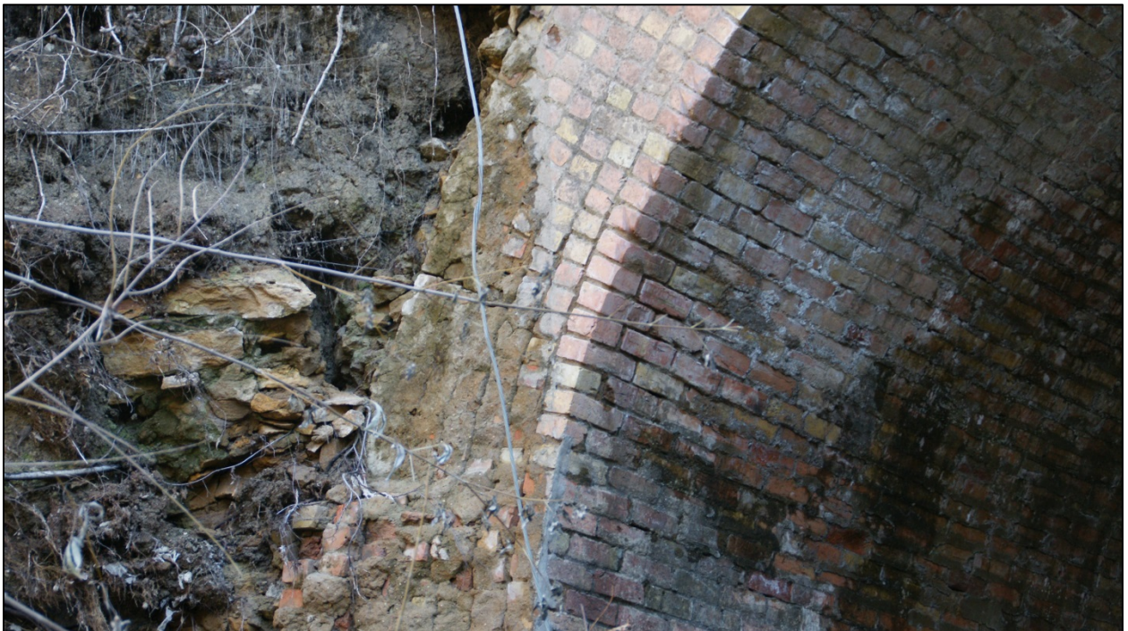
Tension crack near springline of brick arch on left upstream end of culvert.
