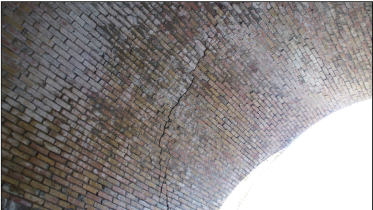
Transverse crack near down stream end of culvert. Runs from crown to footing wall.
