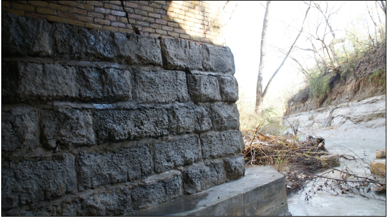
Crack at downstream end of culvert. Runs from brick arch into rock wall and footing.
