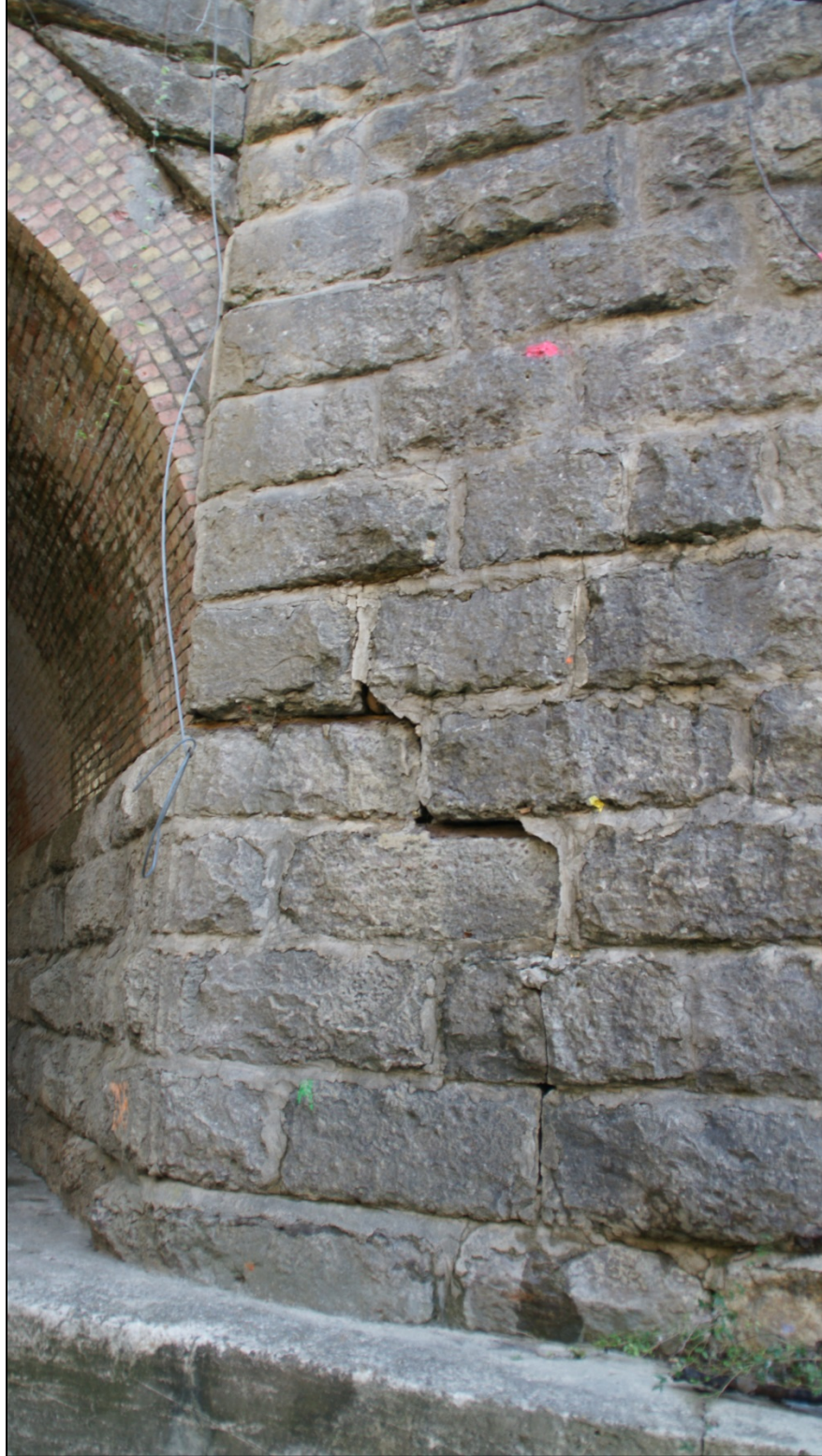
Signs of movement at right upstream wingwall.
