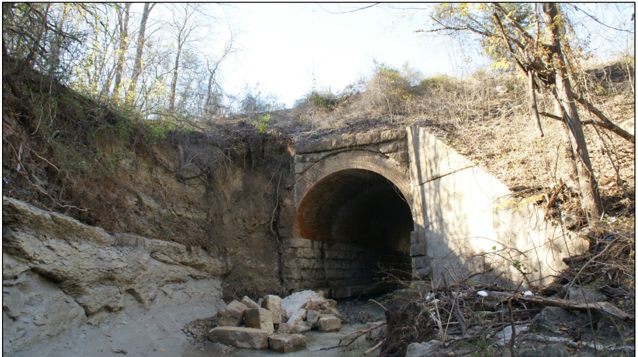
View of downstream end of Brick Culvert. Wingwall fell into creek during the floods the week before. The left downstream wingwall was replaced with reinforced concrete a 1960's flood collapsed the wall.
