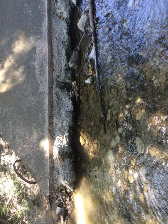
Erosion beneath the bridge
