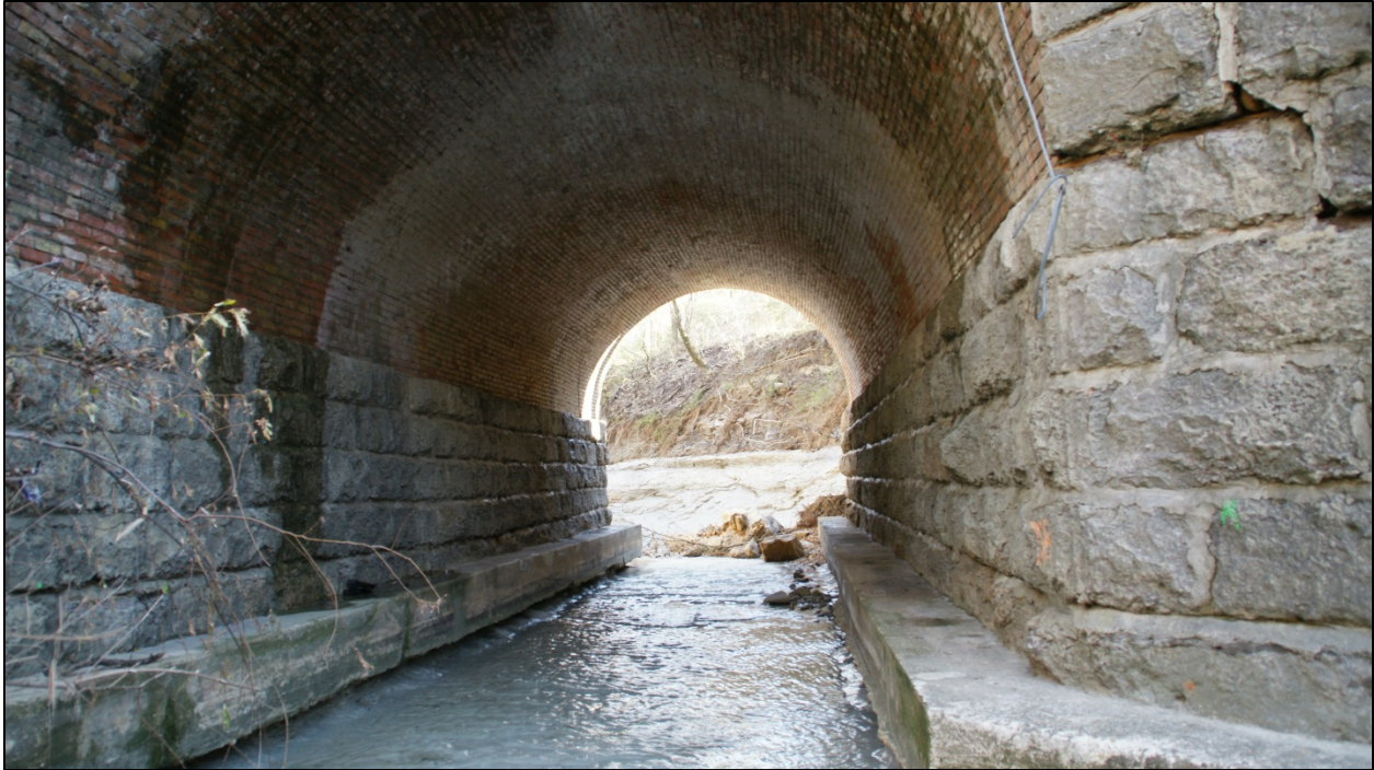
Longitudinal View looking downstream. Note “weeping of brick arch wall.
