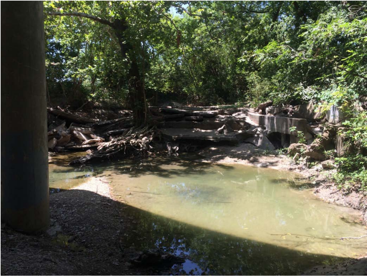
Looking upstream/Collapsed bridge
